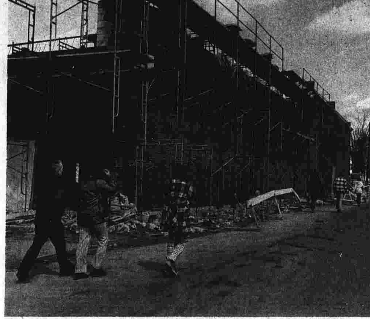
Beginning to take shape is the new gym-library building in the Bennet Junior High School compound. These people are walking along the Wells St. side of the building. Steel, window coverings and other building materials are piled on the second floor waiting to be used. (Herald photo by Pinto)
